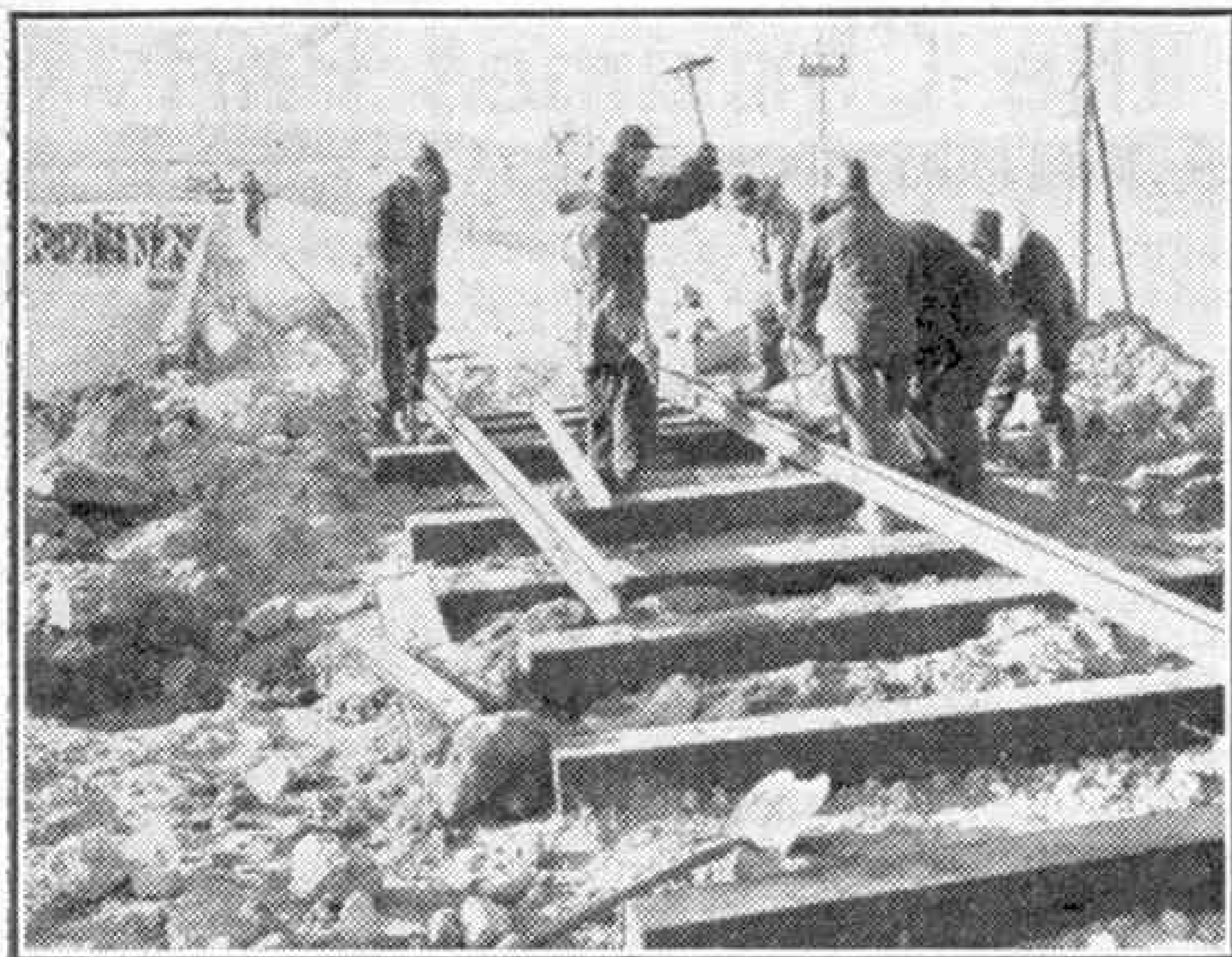
Laying the track of the Labrador railway northward out of Seven Islands towards Burnt Creek, centre of the iron ore fields of Labrador.
