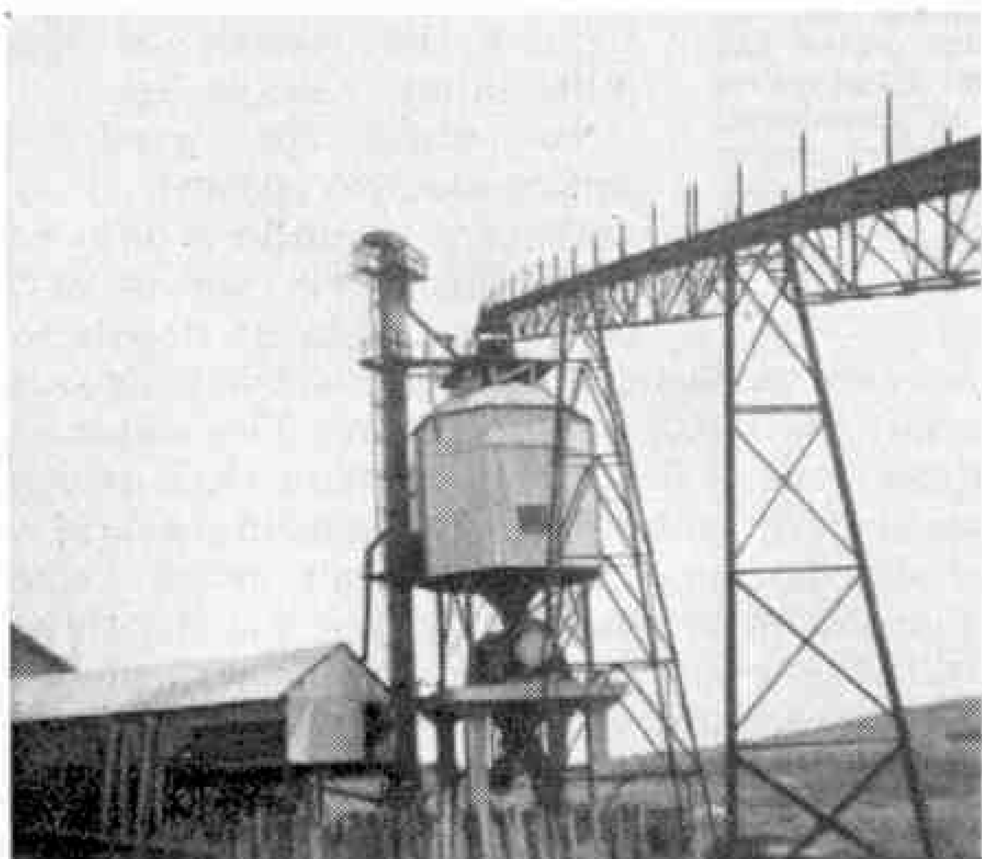
The plant for weighing, batching and mixing concrete. The main conveyor for materials enters at the top, the cement entering through the tube running up the left of the tower.
